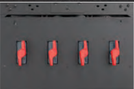
Vacuum zone valves
